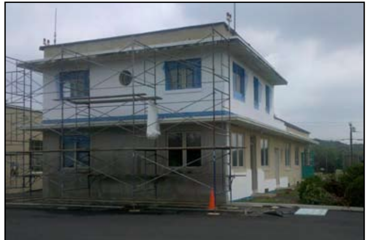
MMKs FBO building gets a facelift with a fresh coat of stucco and a new roof.
