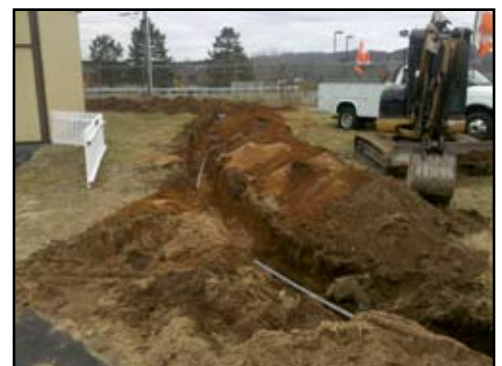
Work is progressing on the ramp lighting at MMK by J E Shea Electric of Plantsville.
