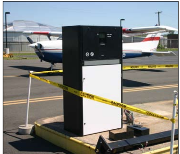
The new self-serve fuel pump being installed at MMK. The old pump has been removed and new piping is being installed between the tank and the pump.
